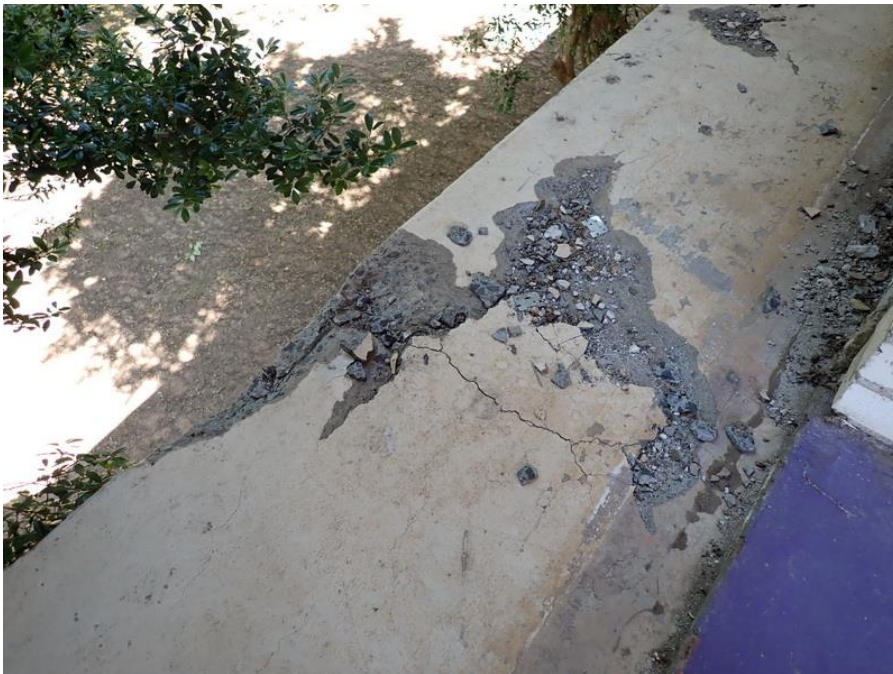
Figure 8. Spalled concrete at edge of Level 4 slab at east facade.
