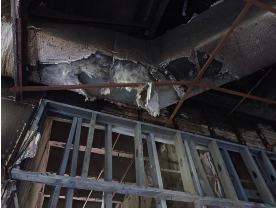
Figure 27. Overall view of interior wall framing that had not burned.
