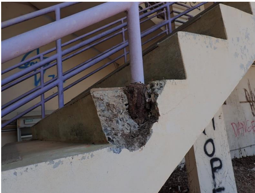
Figure 10. View of typical concrete spall at stair railing post.
