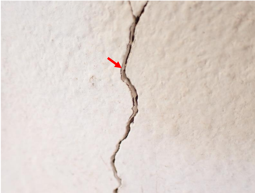
Figure 17. Paint within crack in exterior wall at north facade.
