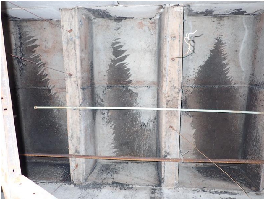
Figure 28. Limited soot staining at underside of intact concrete surfaces above Level 4 fire location.
