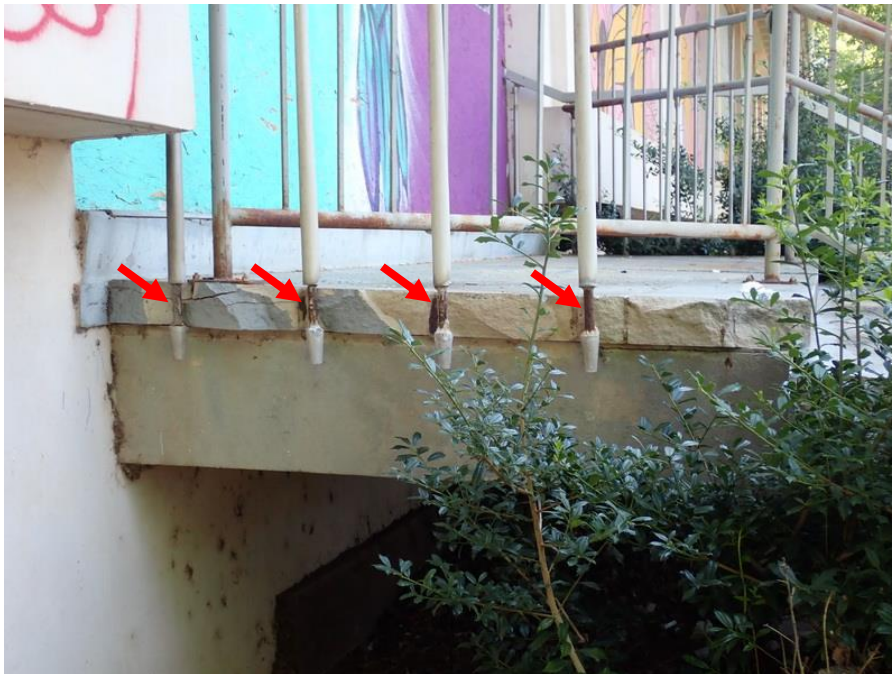
Figure 12. View of spalls along the edge of stair landing at main entrance.
