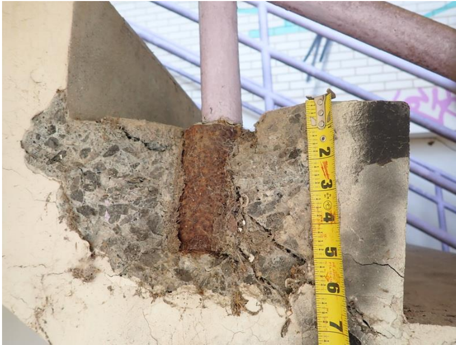
Figure 11. View of typical concrete spall at stair railing post.
