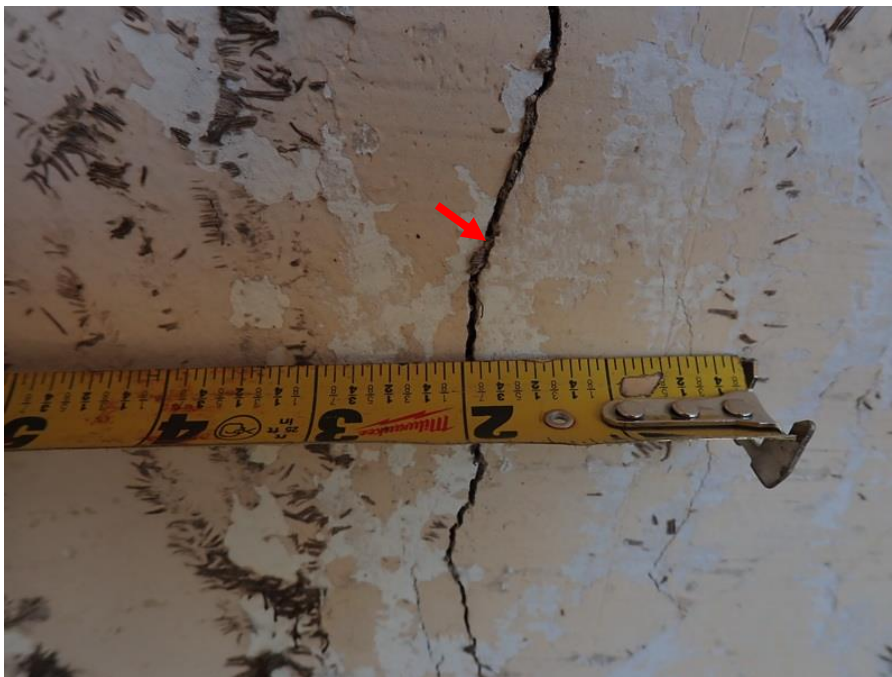
Figure 16. Vertical crack in exterior wall at north facade measures 1/8 inch wide.
