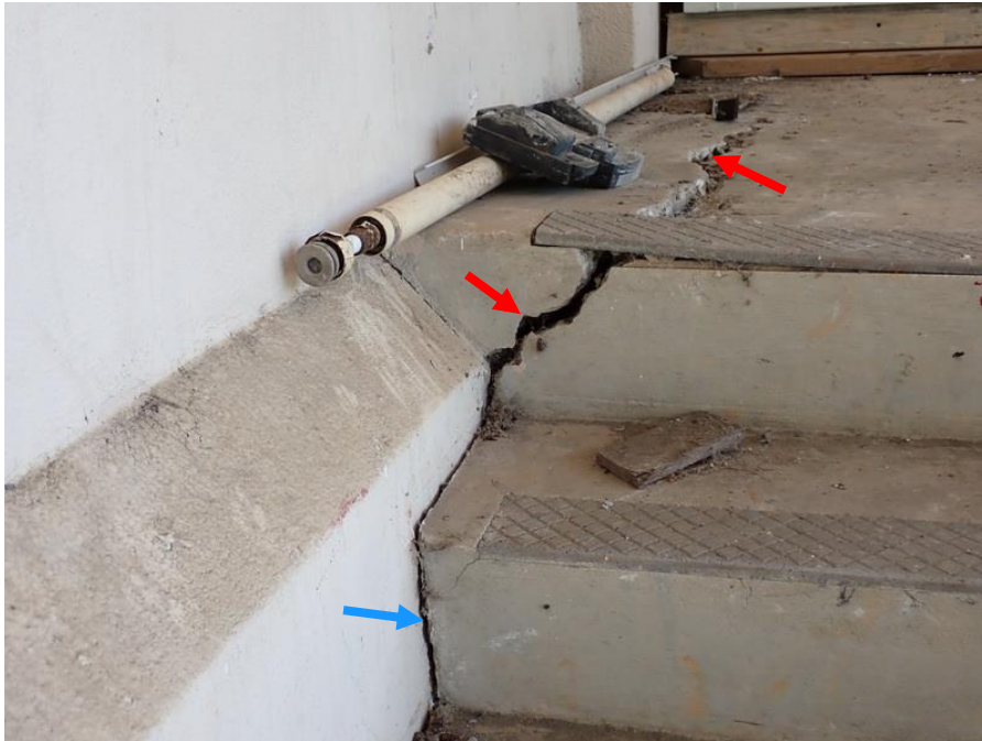
Figure 15. Crack in concrete landing at top of stairs on north facade (red arrow). Joint between north wall and stair treads indicated with blue arrow.
