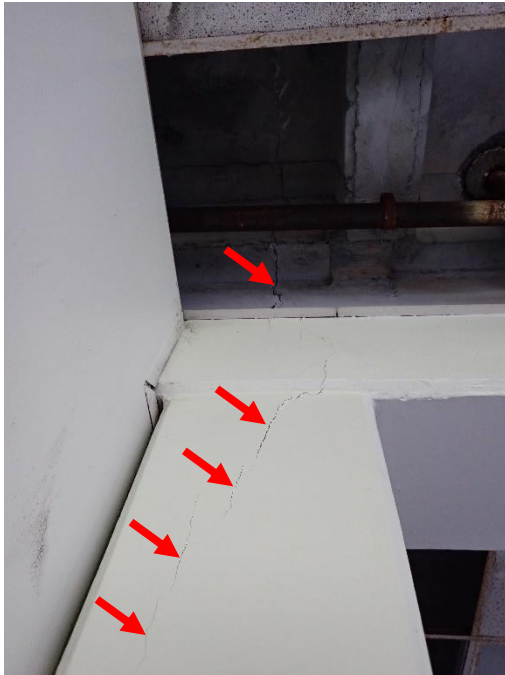
Figure 3. View of vertical cracks in north face of western column at interface with girder.
