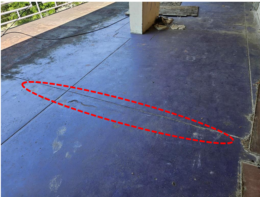
Figure 6. Delaminated areas at Level 4 balcony outlined in red.
