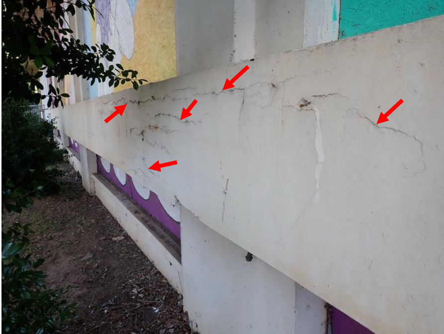
Figure 7. Cracks and delaminated concrete along Level 4 slab edge at south facade.
