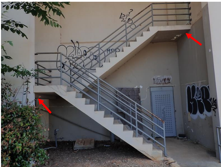
Figure 14. Overall view of the northwest exterior stairway. Locations of edge beam and wall supports indicated with arrows.
