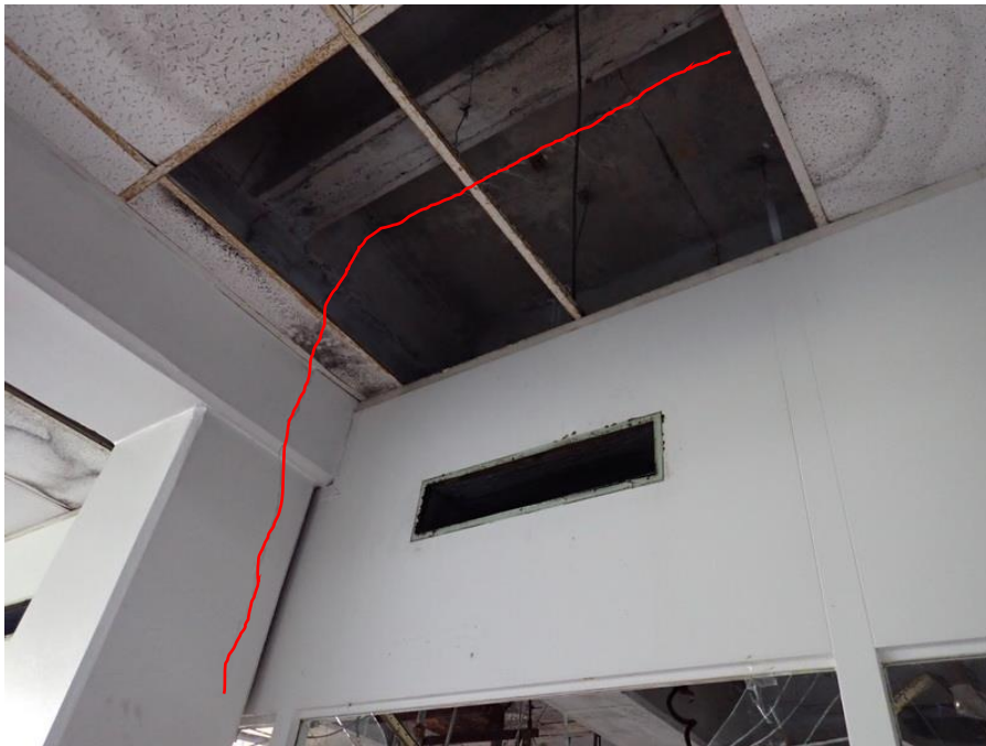
Figure 4. Cracking in western column extending through the floor slab above.
