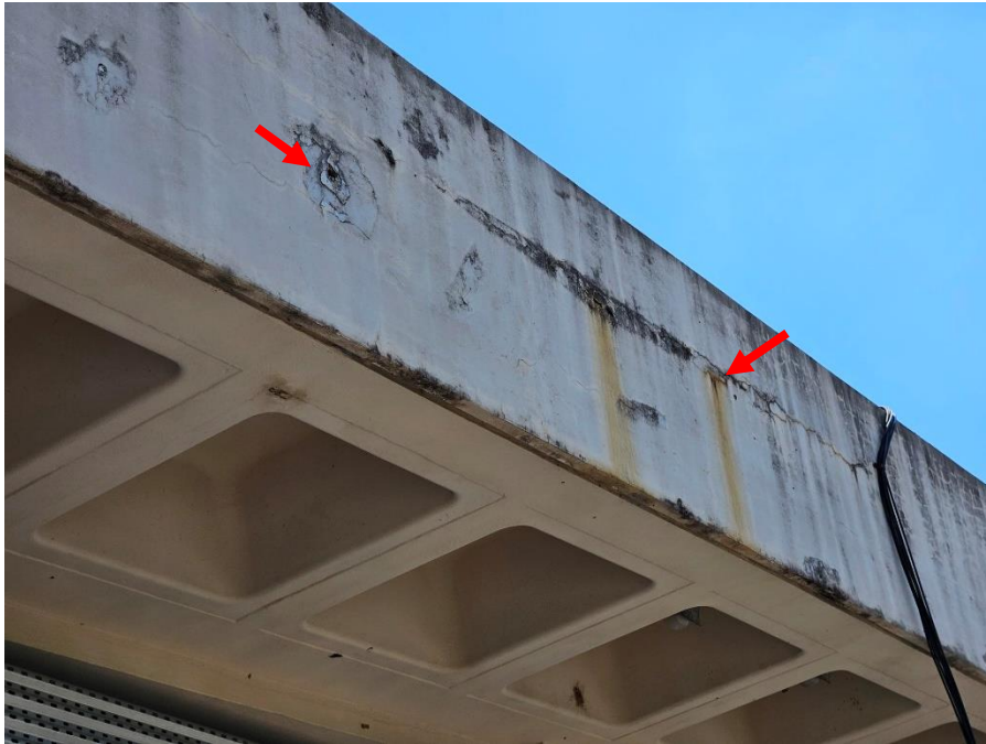
Figure 9. Spalled concrete and corrosion staining at roof edge along north facade.
