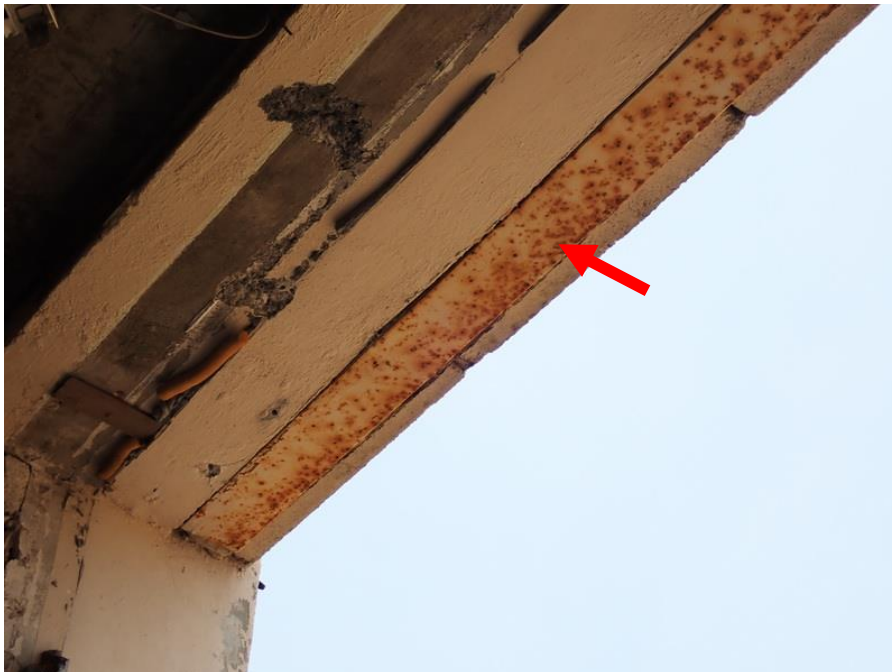
Figure 24. Light surface corrosion on steel lintel support for decorative masonry screen wall at north facade.
