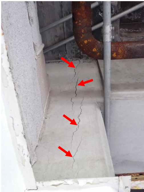
Figure 2. View of vertical cracks in south face of eastern column at interface with girder.
