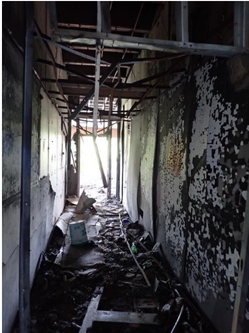
Figure 25. Overview view of interior finishes at location of December 2023 fire on Level 4.
