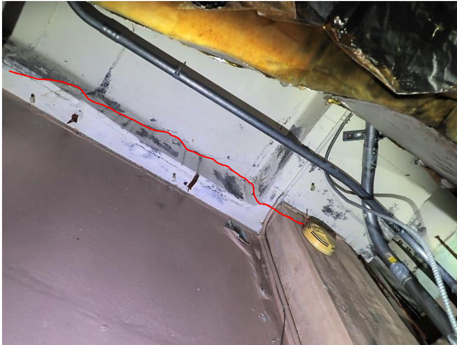
Figure 21. Horizontal crack along edge beam at Level 3 in the south wall.
