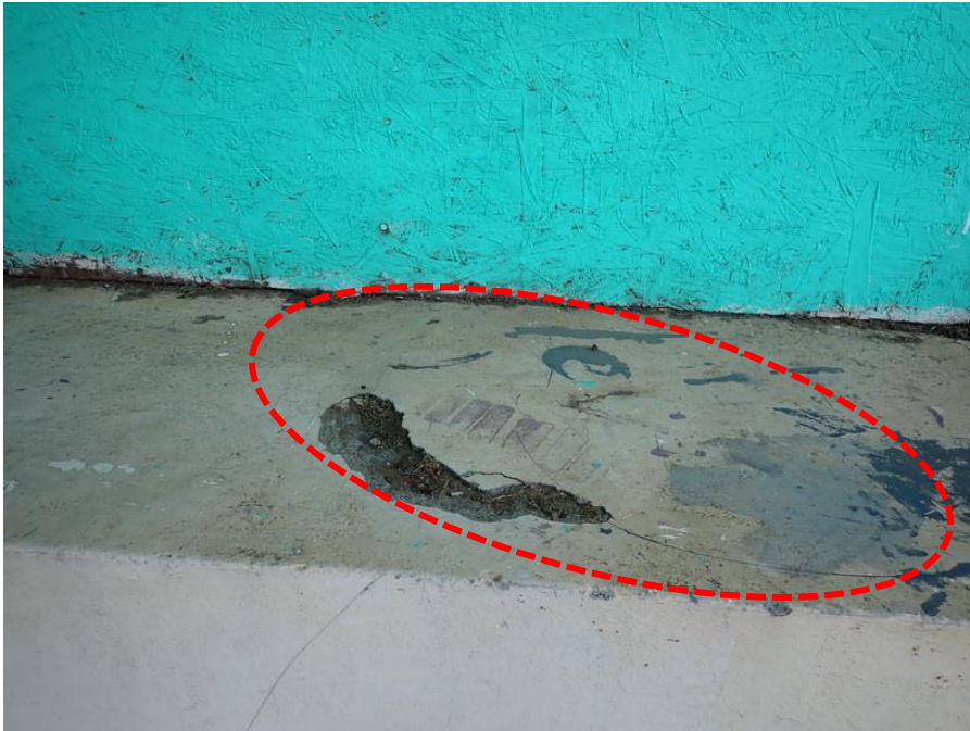
Figure 5. Delamination at top surface of Level 4 slab extension.
