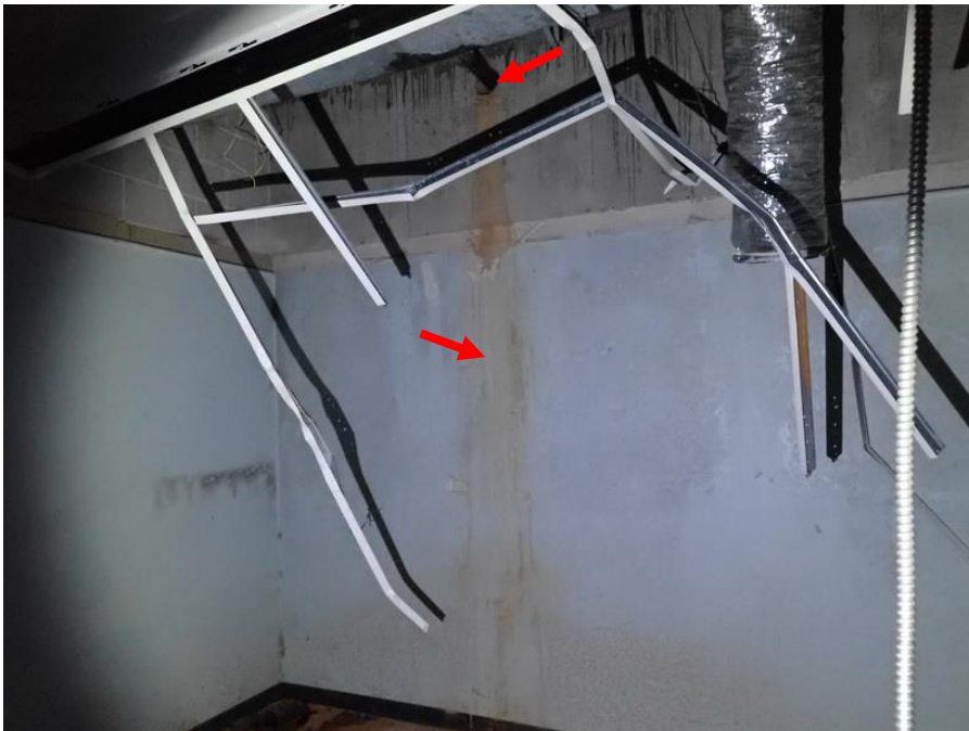
Figure 20. Soil and water staining on south wall beneath pipe penetration.
