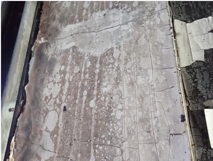
Figure 26. View of crazing in wall finishes in vicinity of fire.
