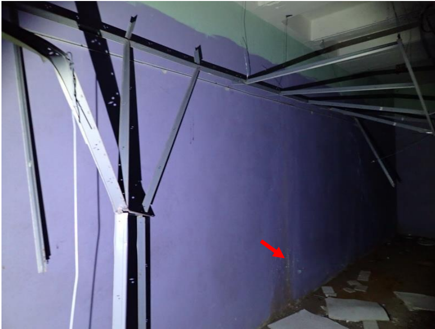
Figure 19. Water staining and bubbled paint at crack in foundation wall.
